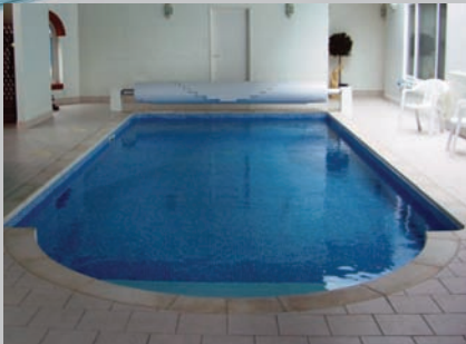
A retrofit above ground system to an existing indoor pool in Buckinghamshire
